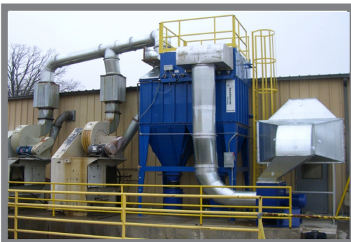
Installed dust removal system.
