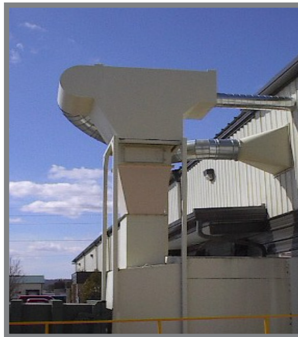
Separator with a return air system and discharge chute into a compactor
