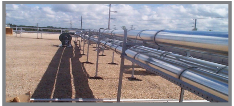
Rooftop installation of blowers, inducers and duct. Long duct runs in a pneumatic system require precise design and engineering to maintain optimal material air flow.
