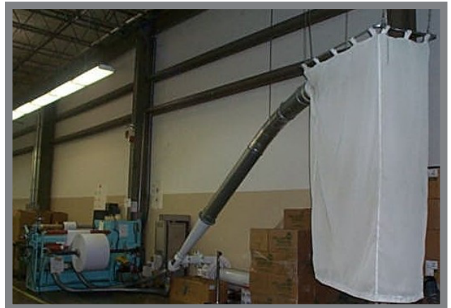
Rented Blower system conveying package for paper trim conveying.
