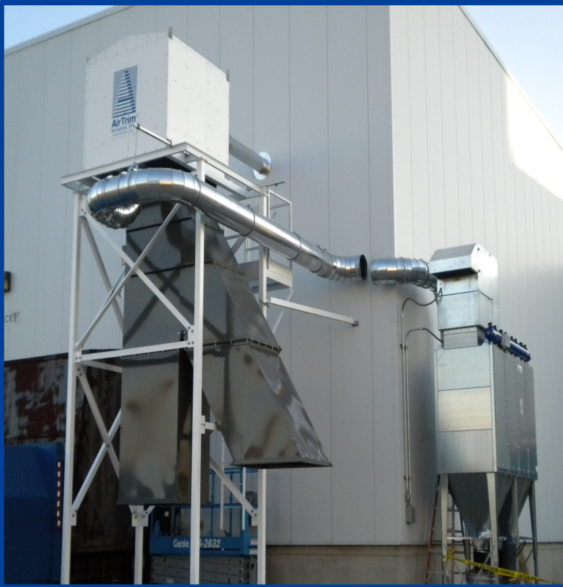
Separator, Diverter Chute and Dust Collector
